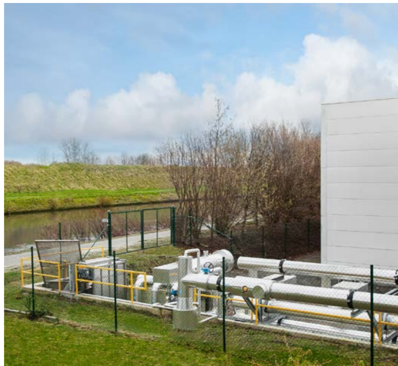
Scheldt Project on plant Avelgem
