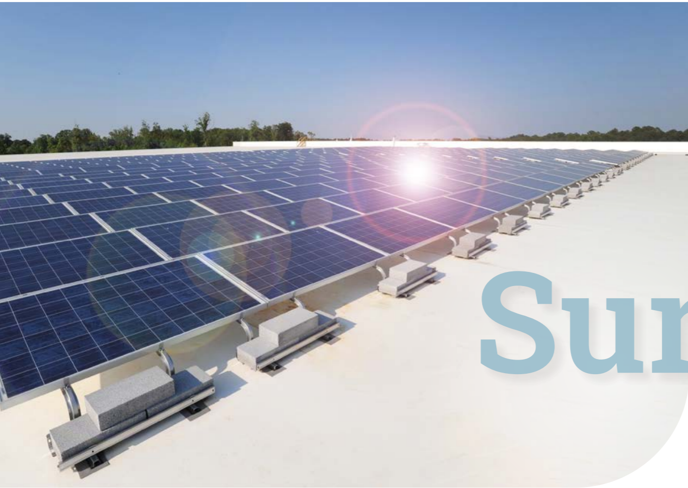
Solar panels on all warehouses
